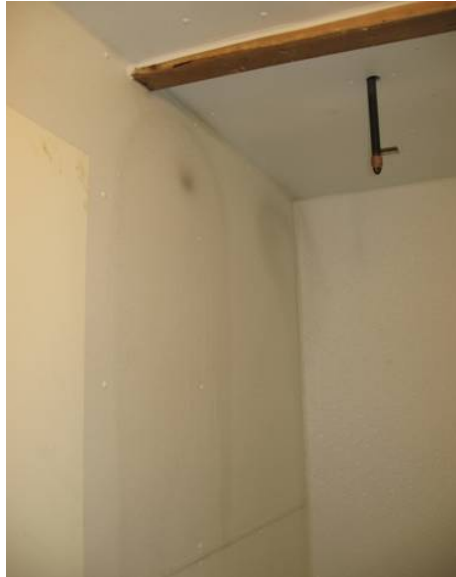
Figure 1. FK-5-1-2 Discharge onto FRP Cladding
