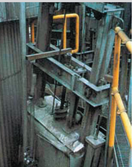
At PNM's sulfuric acid plant, Krytox® keeps knife-gate valves running smoothly at optimum temperatures. Shown here are the valve stem and packing gland.
