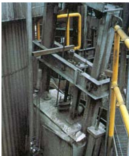
At PNM's sulfuric acid plant, Krytox® keeps knife-gate valves running smoothly at optimum temperatures. Shown here are the valve stem and packing gland.
