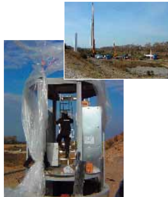
Mistral Energie's 1000 kW Vestas V52 wind-turbine in construction at Port-Saint-Louis-du-Rhône. With the help of NOMEX® thermal protection, the size of the Pauwels SLIM® transformer was reduced, so that it could be installed in the tower.
