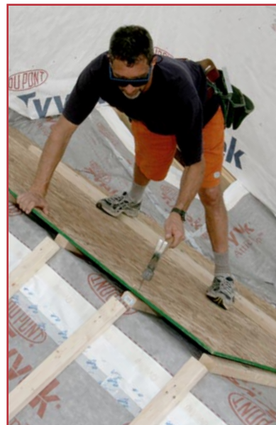
Install sheathing with air slot at least 1½ in. wide at ridge
