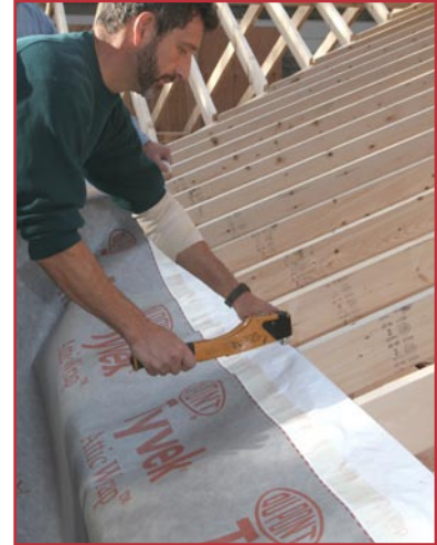
Align Tyvek® AtticWrap™ to chalk line and fasten to the tops of the rafters
